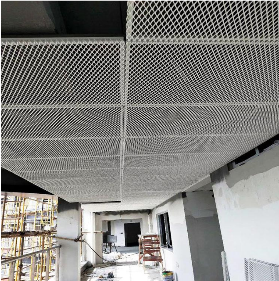
Ceiling installation: welding the Expanded Metal Mesh to the frame then install the frames
